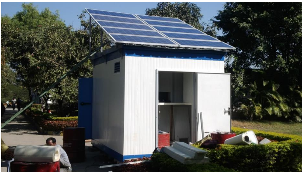
Small Cold-store with Solar Panels for captive use.
