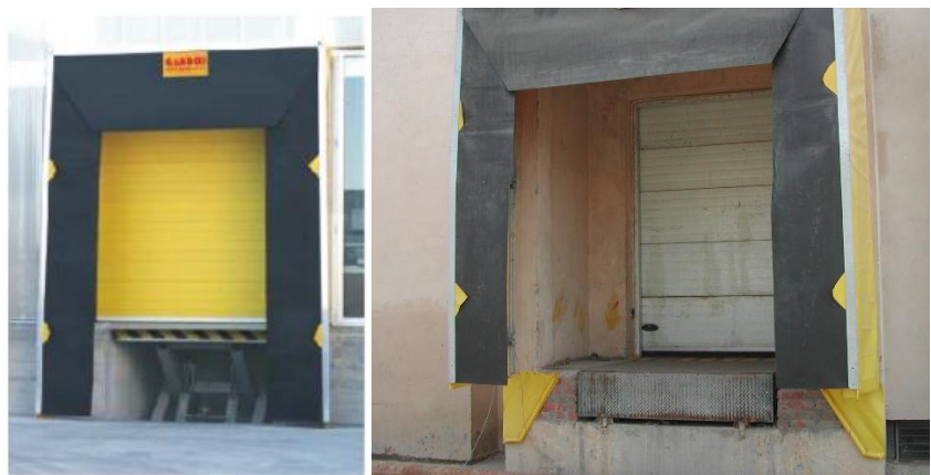
Sheltered dock with leveller and insulated Door
